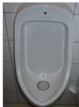
Figure 2: Waterless urinal (Source: A. Rechenburg)
