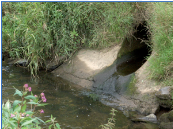
Figure 1: Discharge of treated sewage leaving the STP
