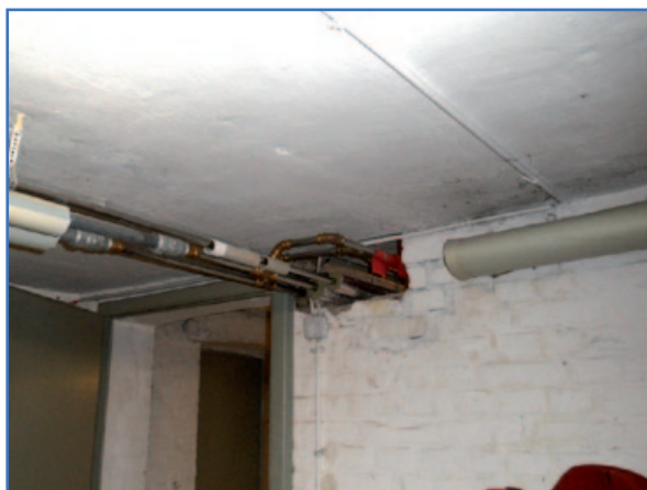
Figure 2: Insufficient insulation of the piping Source: IHPH
