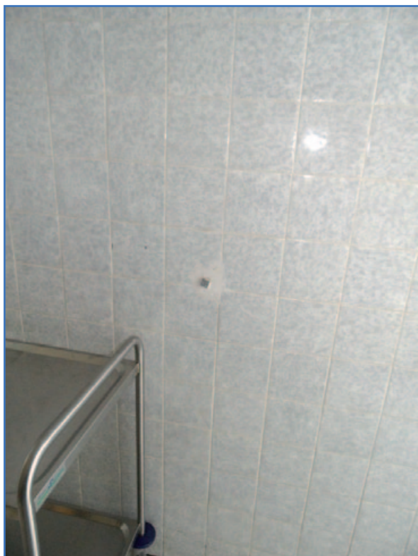
Figure 4: Dead pipe end Source: IHPH
